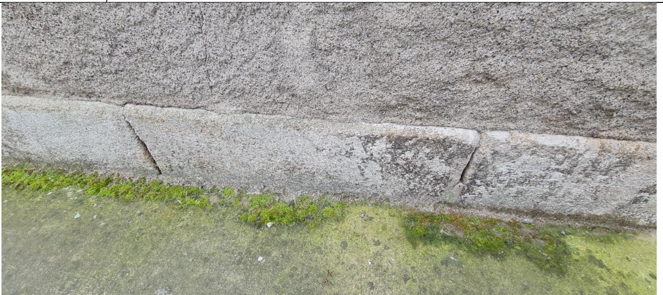
Fig. A20 Detail of granite plinth at base of east façade (onto Bow Street)
