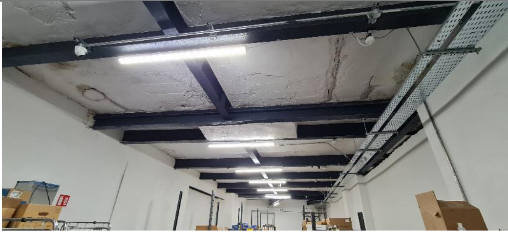
Fig. A40: Interior of warehouse off Bow Street, on east side of site
