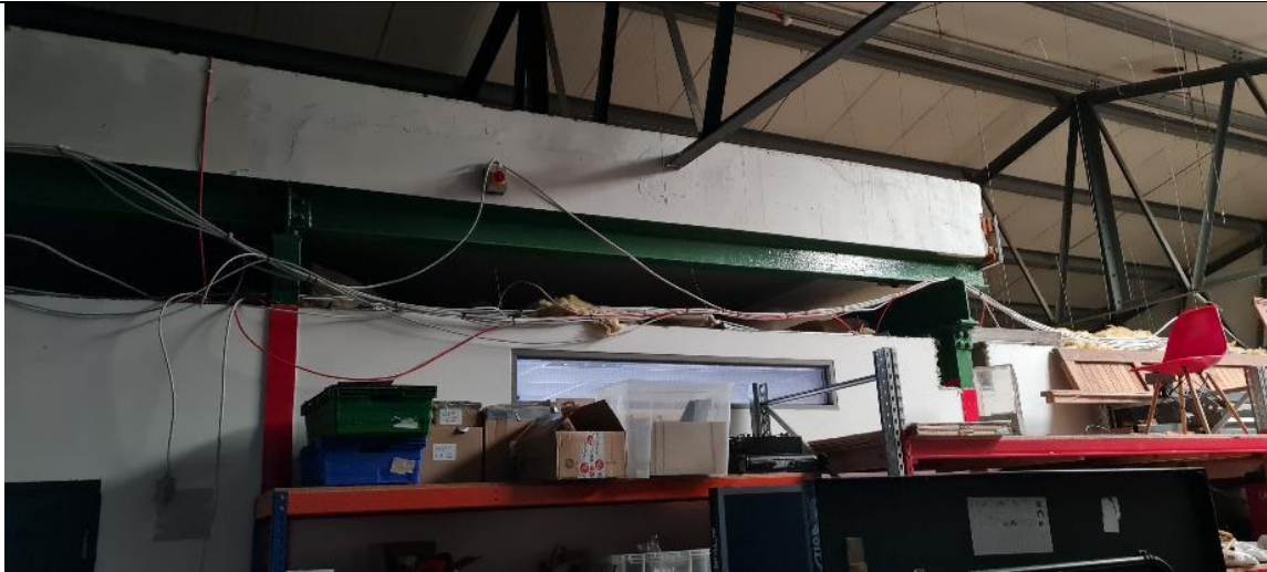
Fig. A54 Modern metal deck roof on steel trusses over first floor storage area within microbrewery. Note: 1920's steel frame (painted green) does not support roof structure.
