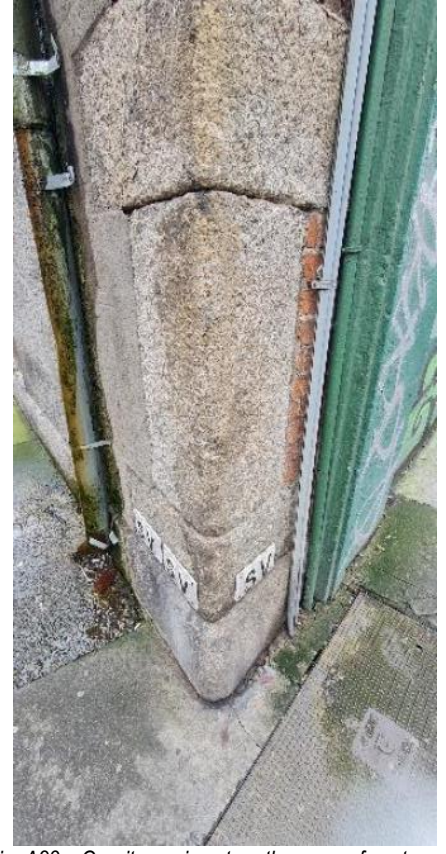
Fig. A23: Granite quoins at north corner of east façade (Bow Street)
