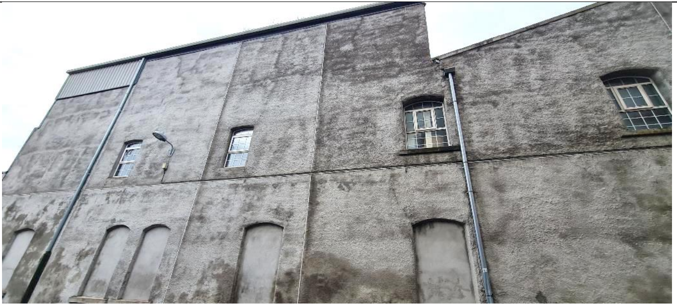
Fig. A18 Detail of southern part of east facade onto Bow Street.
