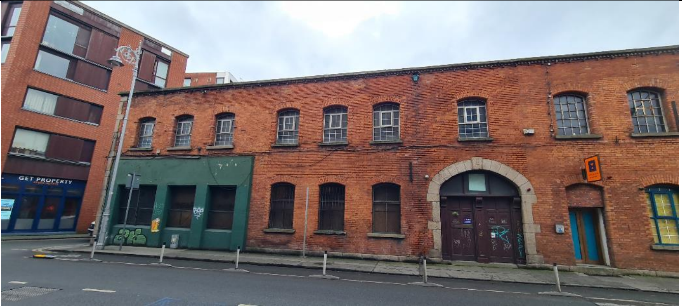
Fig. A1 Eastern end of front (north) façade onto North King Street. This section of façade dates from c.1885
