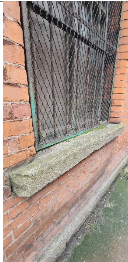
Fig. A6: Detail of granite window sill at east end of front (north) facade
