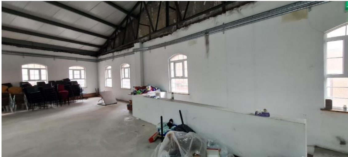
Fig. 16 First floor interior, looking towards the north-east corner of the site. There are surviving segmental arched window openings on both the north (left) and east (right) external walls. The gable and roof structure are clearly of much later date.
