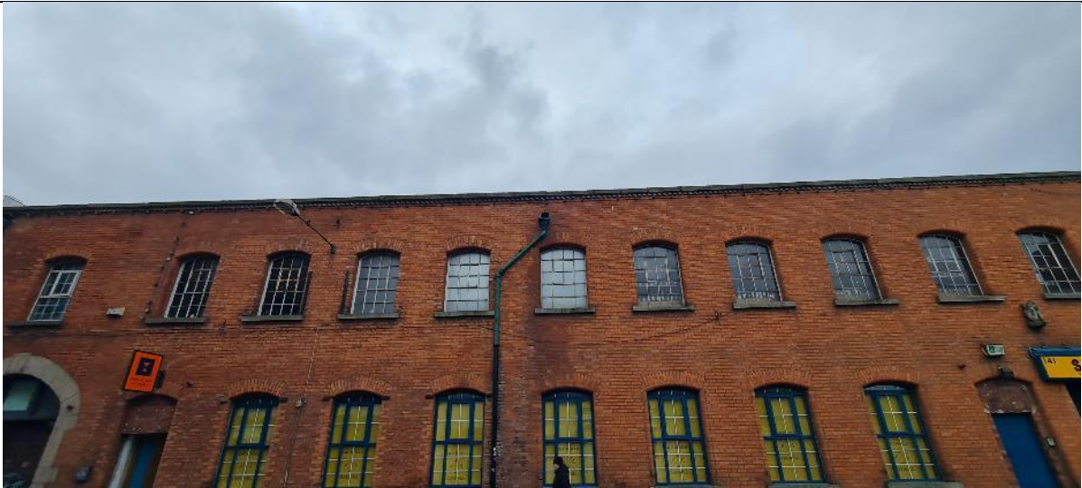
Fig. A4: Surviving steel frame windows at first floor level in central section of front (north) facade
