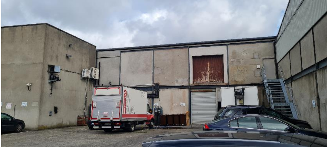
Fig. A24: Goods yard to rear of 139-149 North King Street – south façade of two-storey block on north side of yard
