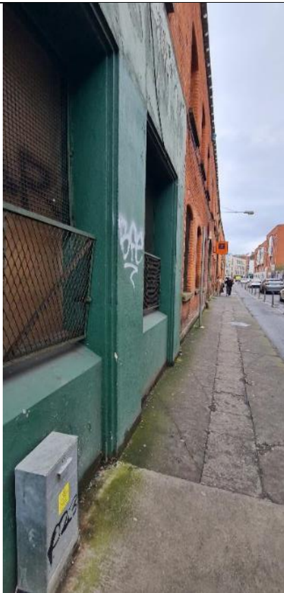
Fig. A5: Detail of shopfront at east end of front (north) facade
