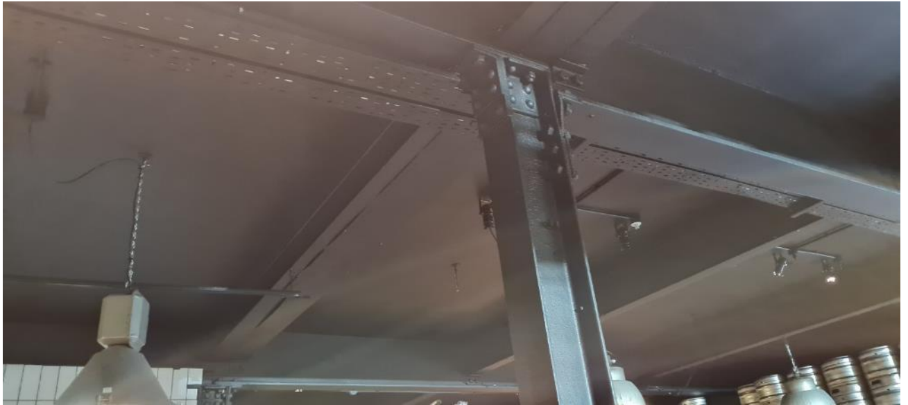
Fig. 19 Interior of micro-brewery (ground floor level), showing interface between retained 1920's steel column and modern ceiling/floor slab.
