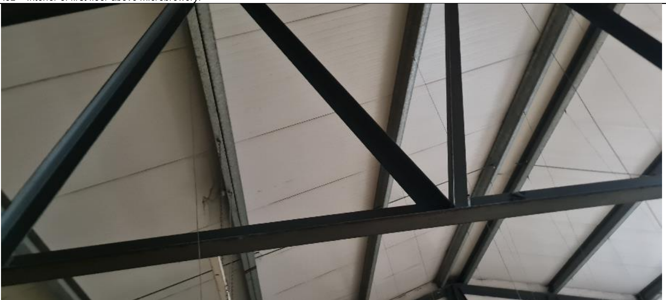
Fig. A53 Modern metal deck roof on steel trusses behind suspended ceiling of first floor above microbrewery
