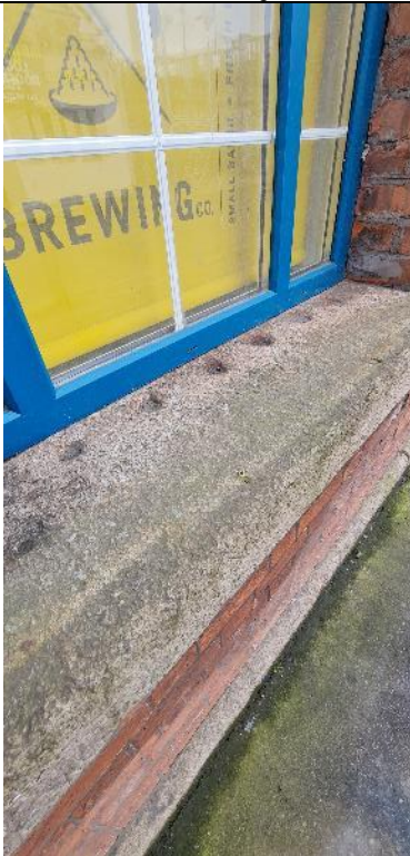
Fig. A9 Detail of window sill on east part of façade (c.1885)
