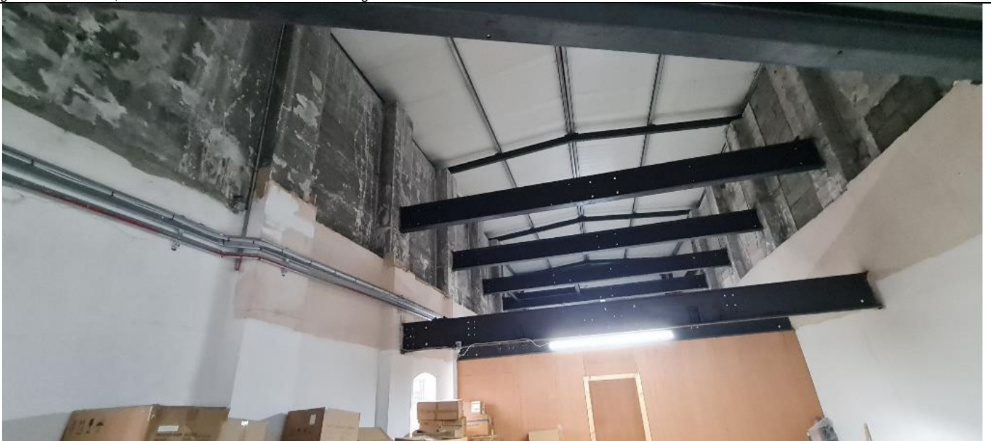
Fig. A61 First floor, with east external wall (to Bow Street) on left
