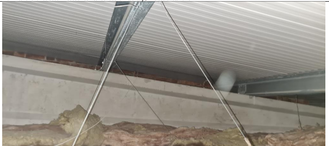
Fig. A47 Soffit of metal deck roof above suspended ceiling over first floor of 'Little Italy', wholesale retail unit
