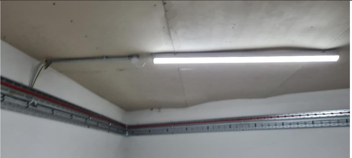
Fig. A66 Interior of basement – curved surface of plasterboard lining to ceiling is a possible indicator of a shallow vault overhead
