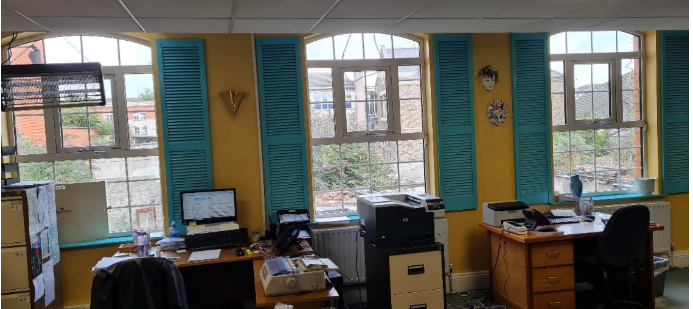
Fig. A45 Windows on north external wall of office accommodation at first floor above 'Little Italy', wholesale retail unit
