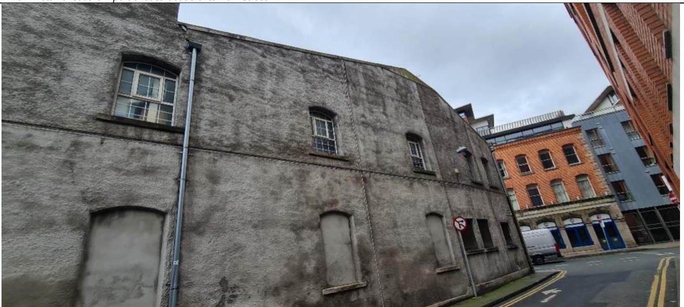
Fig. A19 Detail of northern part of east facade onto Bow Street.
