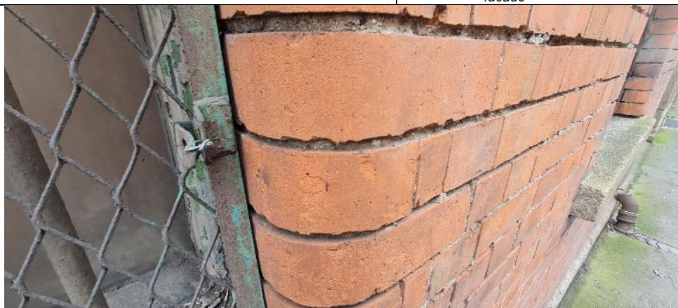
Fig. A7: Detail of rounded brick reveal to ground floor window opening at east end of facade
