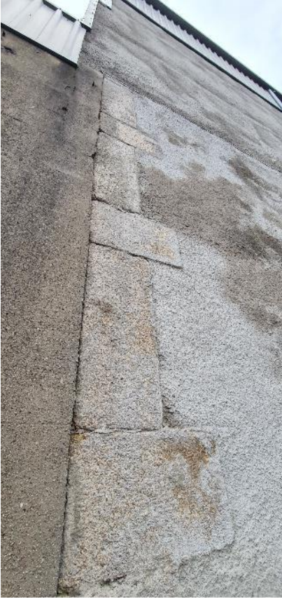
Fig. A21: Granite quoins at southern end of east façade (Bow Street)
